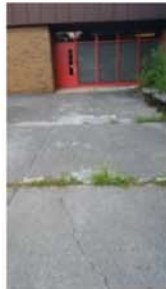
GLE, FBE, HAE Replace concrete sidewalks (also add a sidewalk at HAE)
