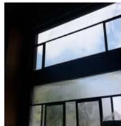
BEL Replace fogged window panes
