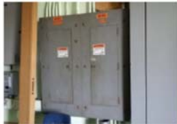
Electric Panel Strategic Replacements CMS, GLE, BEL, MBE, SMS
